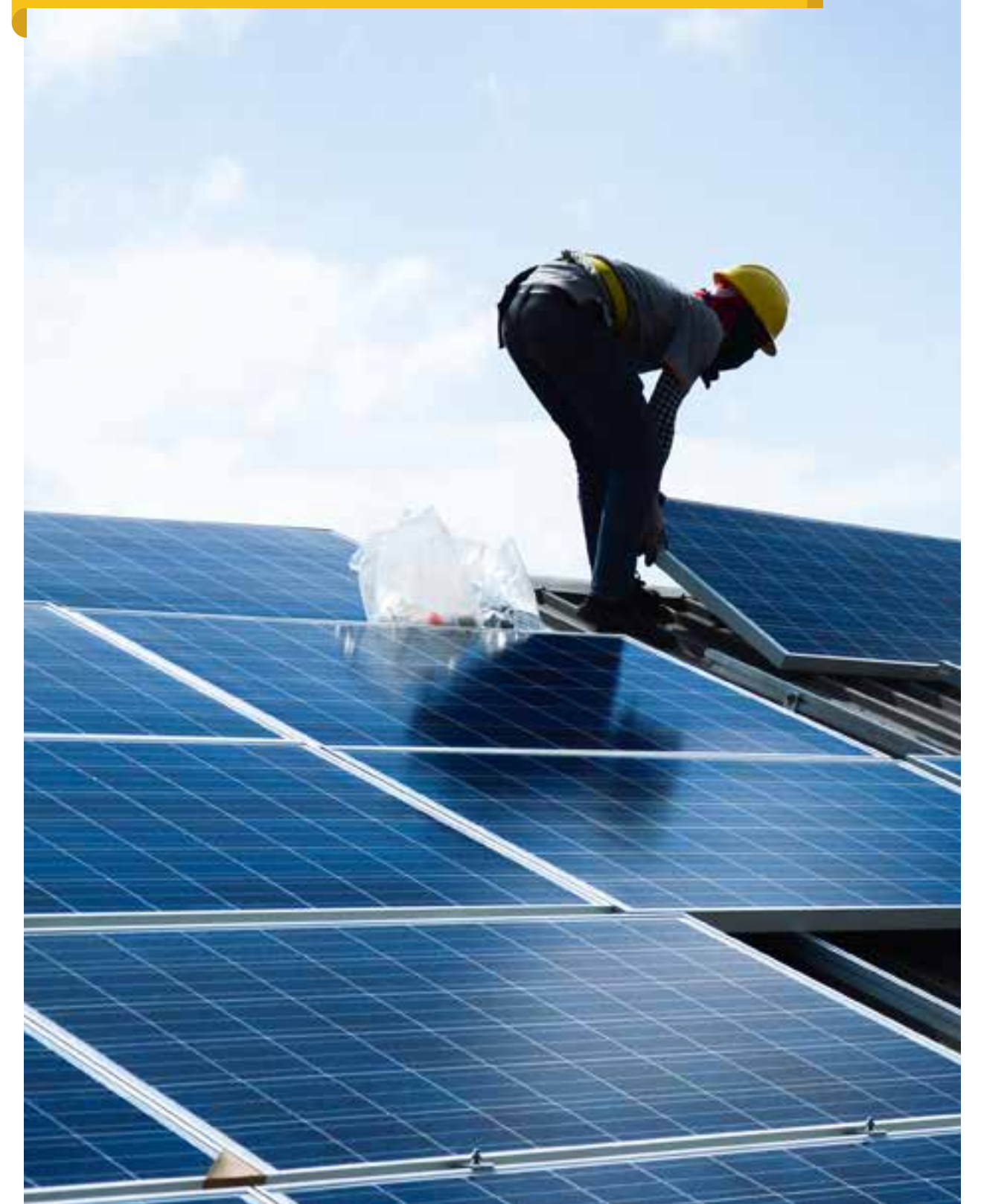
Roof spaces used for photovoltaics
