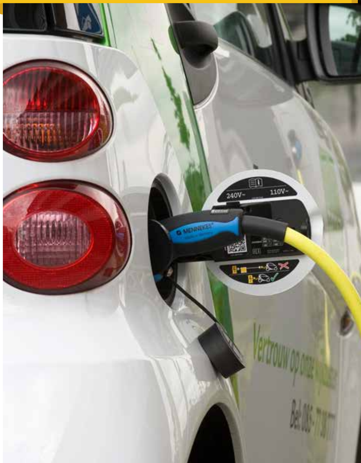
Electric car parking and charging points
